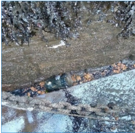
Sewage solids (Image: South West Water)
