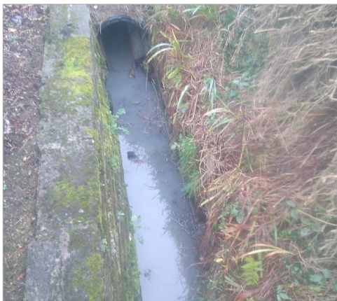
Grey coloured water (sewage smell) (Image: South West Water)
